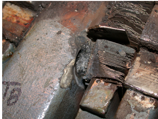
Failure due to Loose Step Iron
