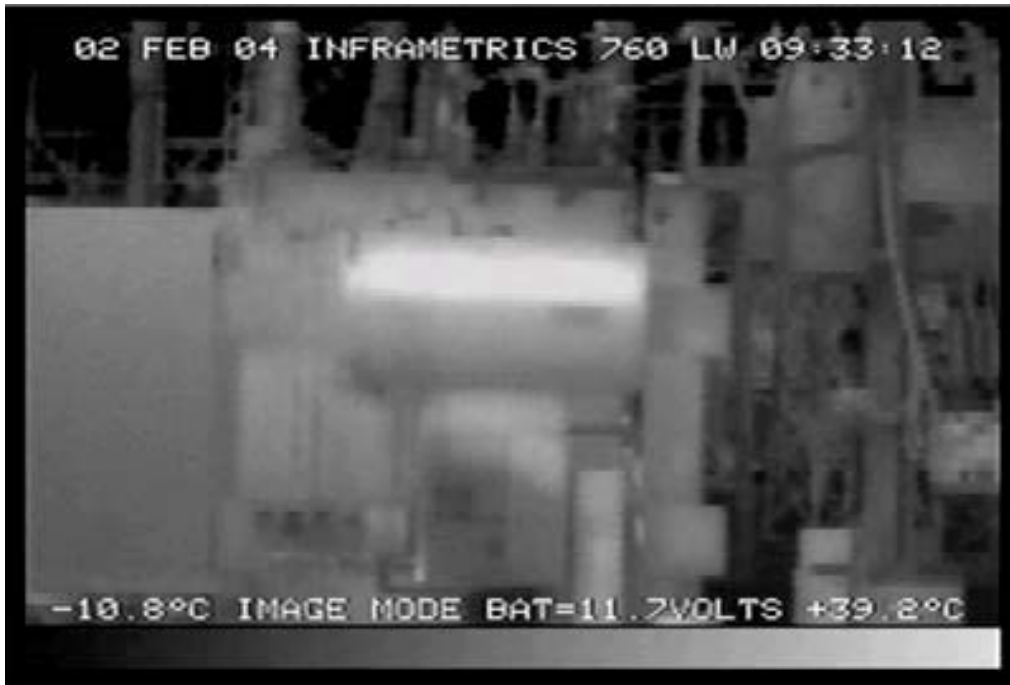
Infrared Image of Transformer with Problem McGraw Edison 550C LTC FIGURE 7
