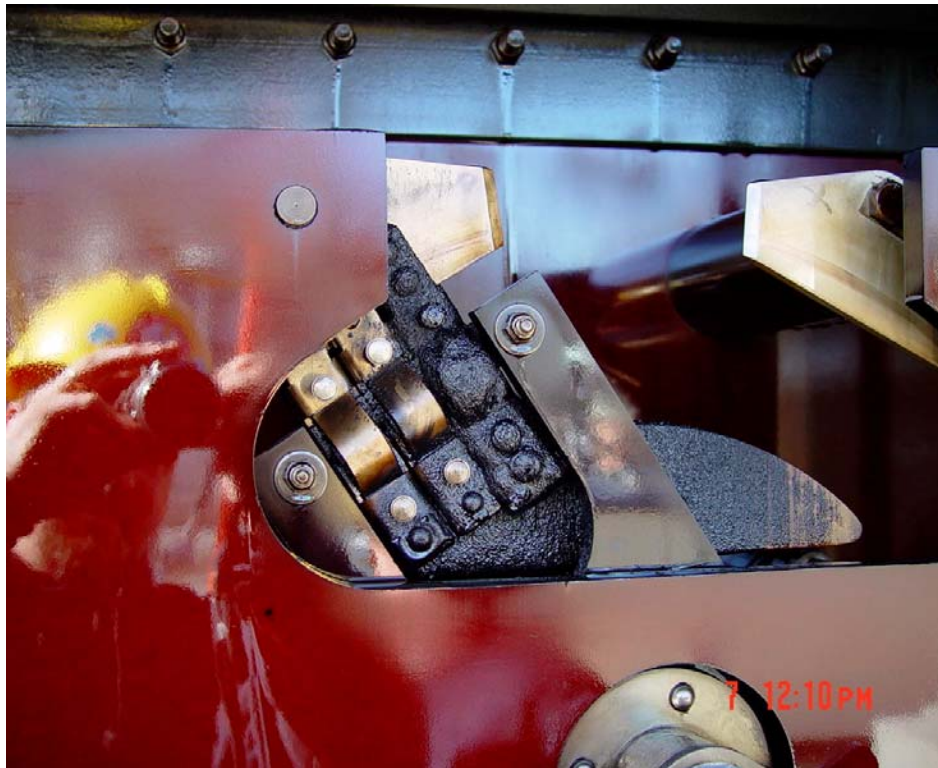
Close up of McGraw Edison 550C LTC with Coking on Reversing Switch FIGURE 9
