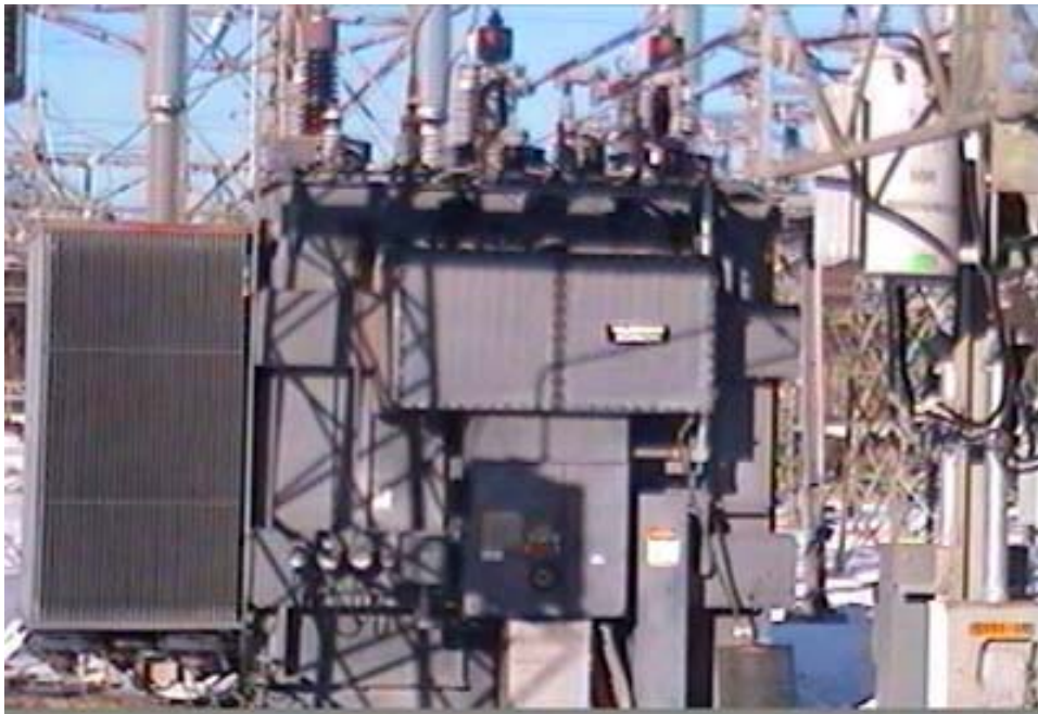
Photograph of Transformer with Problem McGraw Edison 550C LTC FIGURE 6
