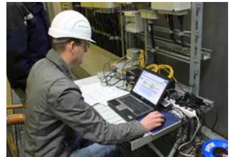
Rotating Machine Partial Discharge Measurements using 80-pF Line Couplers
