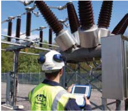
On-line substation partial discharge survey using Doble PDS100.
