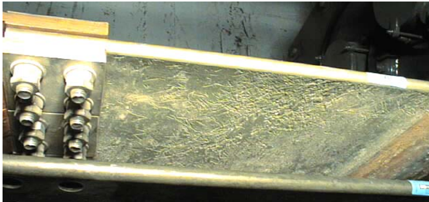
FIGURE 1 Corroded Bus Bar Surface
