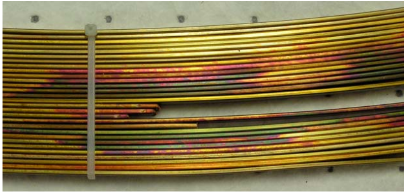
EVIDENCE OF COPPER SULFIDE, PURPLE, GREEN, BLUE AND GREY DISCOLORATION OF CONDUCTOR FROM TRANSFORMER WITH FOUR YEARS OF SERVICE FIGURE 1
