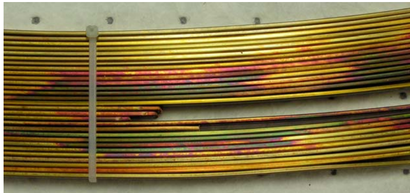
Evidence of Copper Sulfide, Purple, Green, Blue and Grey Discoloration of Conductor FIGURE 1
