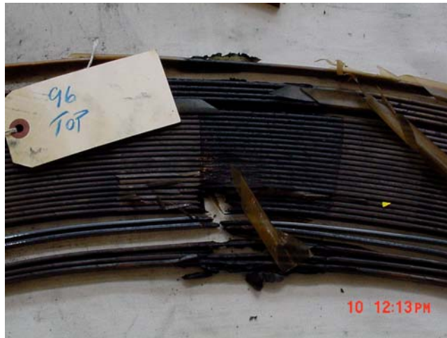
Evidence of Discharge Activity on Disk from Failed Transformer FIGURE 2
