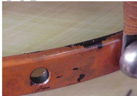
Figure 2c: Remaining Copper Sulfide that was Flaking off on Ring Around the Diverter Switch Compartment
