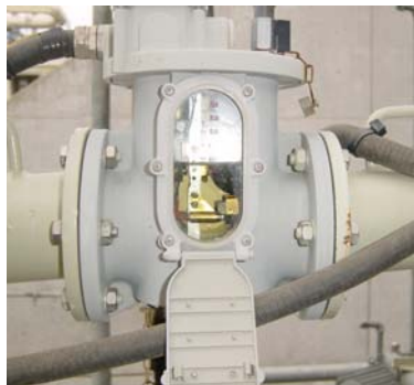
Picture of Bucholtz Gas Relay (Found half filled with Gas)
