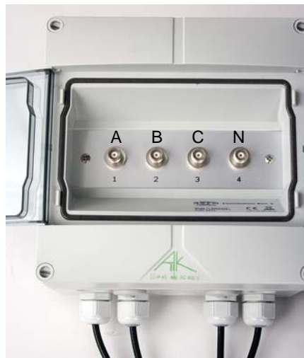
Figure 9 Connector Box Labeled A, B, C, N
