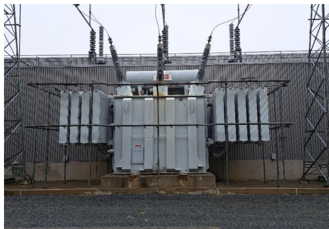
Transformer T1 Figure 3
