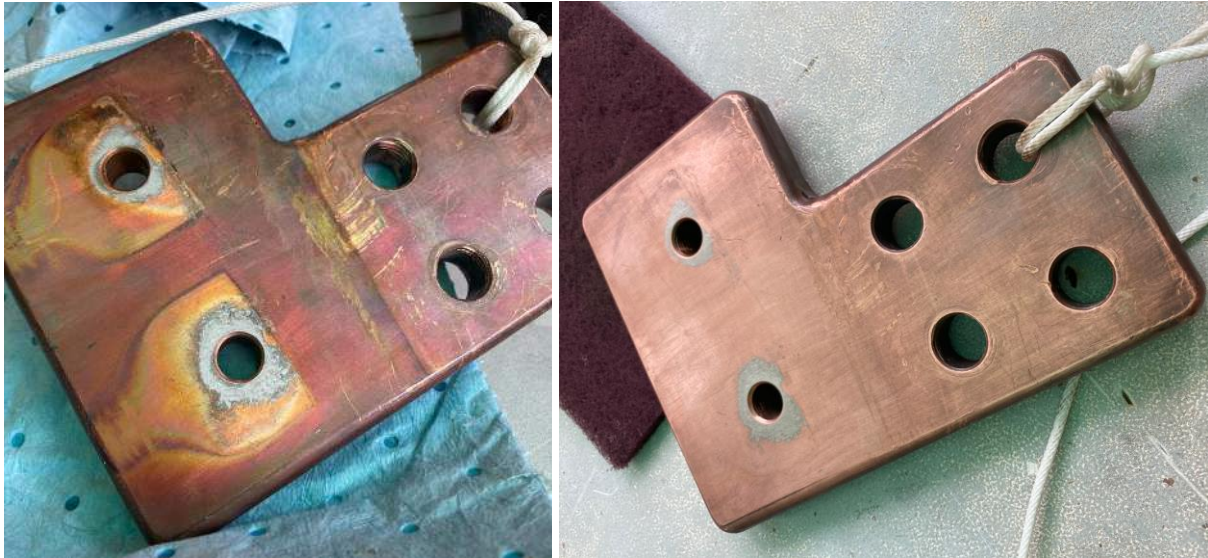
Copper Connection Plate (Before and After Cleaning) Figure 8
