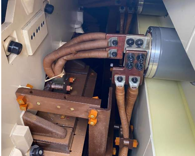
Winding Leads Connected to the Copper Plate at the Bushing Figure 7
