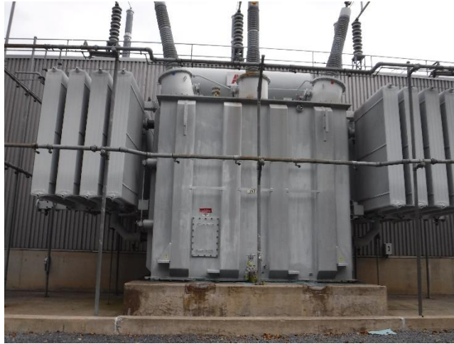
Transformer T2 Figure 4
