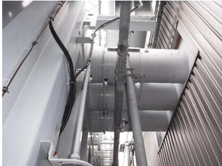
Insulated Phase Bus Duct Figure 5
