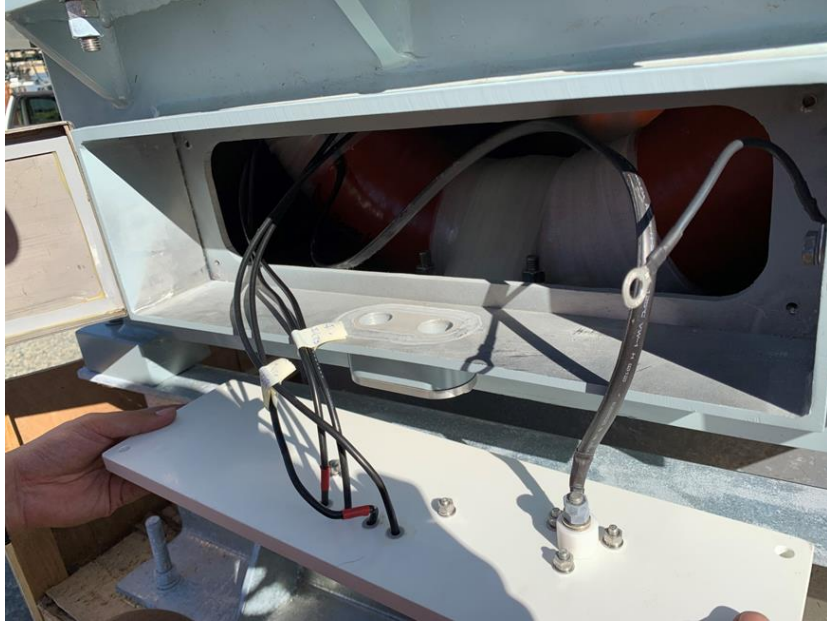
CT Terminal Box Figure 10
