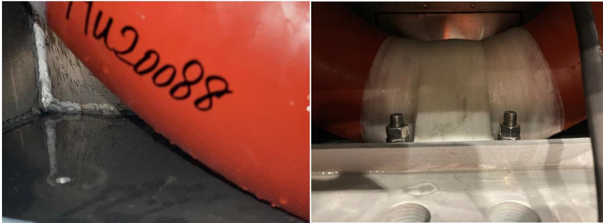
CT Internal Wet Condition Figure 3
