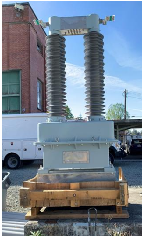
Site Testing CT Figure 9
