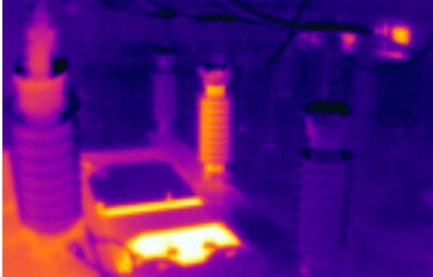
Thermal Snapshot Showing Arrester Heating During Open-Delta Situation Figure 21
