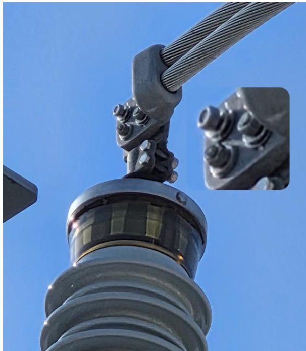
Image Showing Loose Bolted Connection on Bushing Pad Figure 16
