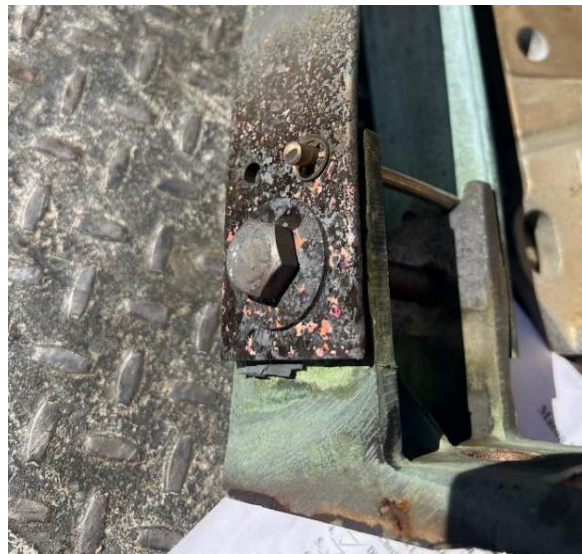
Image Detailing Damage on Monitored Switch Figure 24
