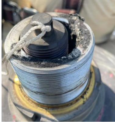
Physical Damage to Bushing from Arcing Figure 10
