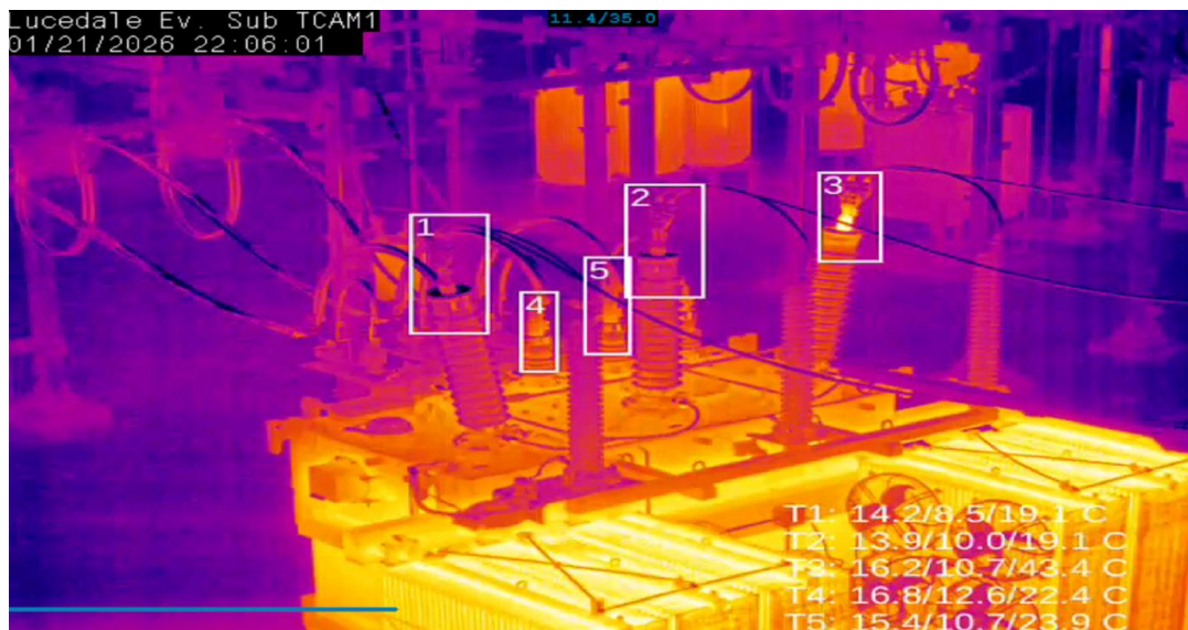
Thermal Image Showing 20°C Delta Between High-Side Bushings Figure 35
