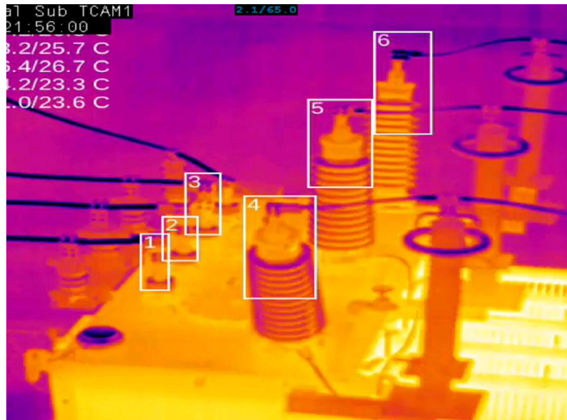
Thermal Image Showing Low-Side Bushing Temperature 25.7 °C before Load Increase Figure 25
