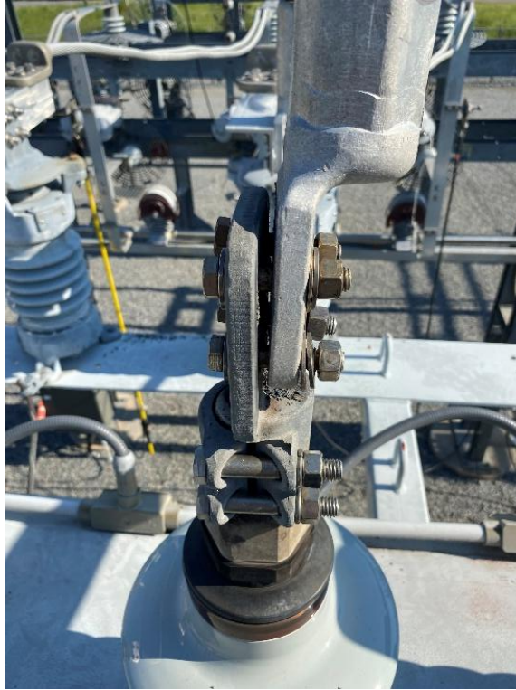
Image Showing Loose Connection and Damage Figure 19
