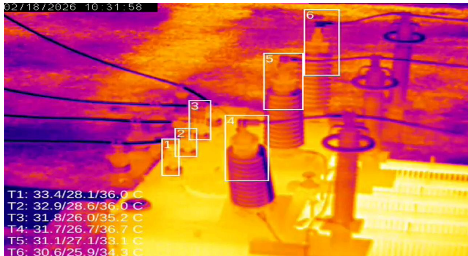
Thermal Image Showing Bushing Temperatures after Repair Figure 29
