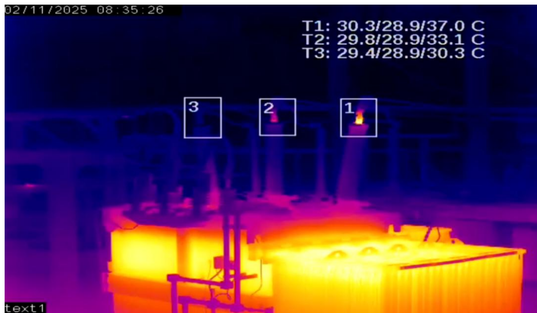
Thermal Image Showing High-Side Temperature Delta During Commissioning Figure 32
