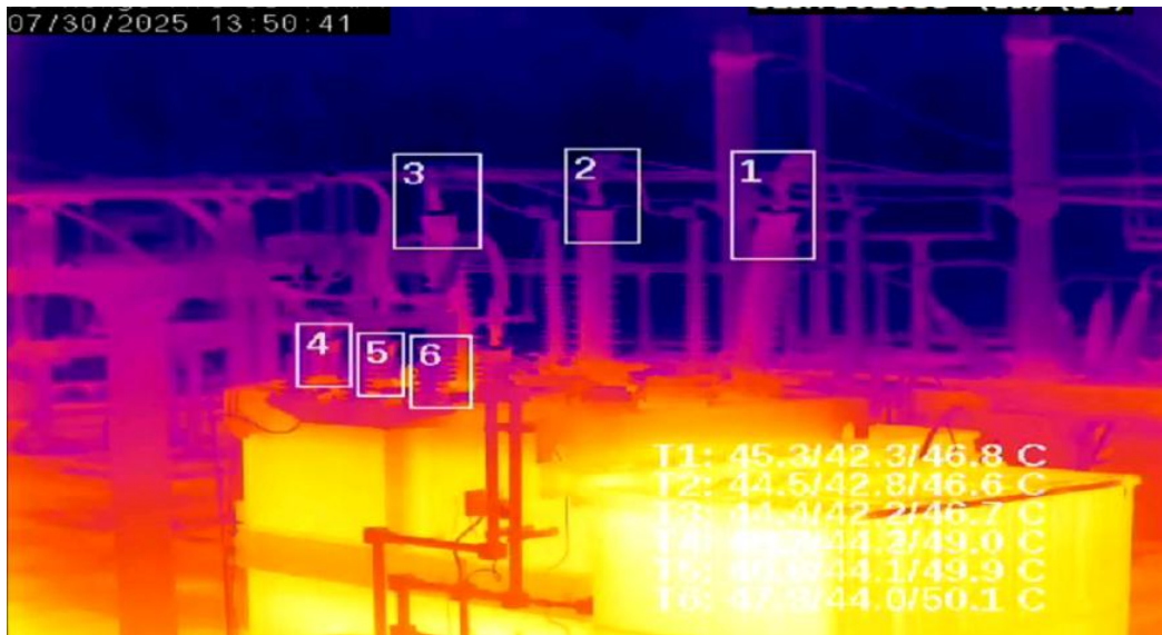
Thermal Image 5 Months after Repairs with No Temperature Delta Figure 34
