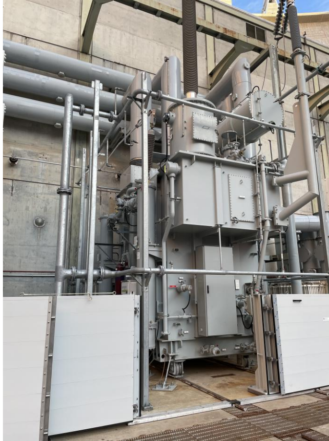
Transformer Fire Protection and Secondary Fluid Containment Systems Figure 5
