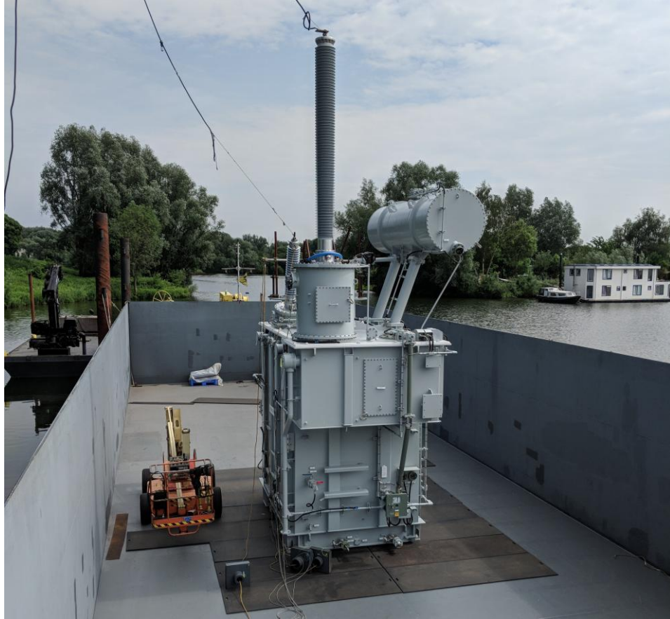
Prototype Transformer in Short-Circuit Test Configuration Figure 6
