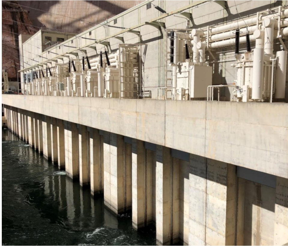
Transformer Deck at Site 2 (2016)
