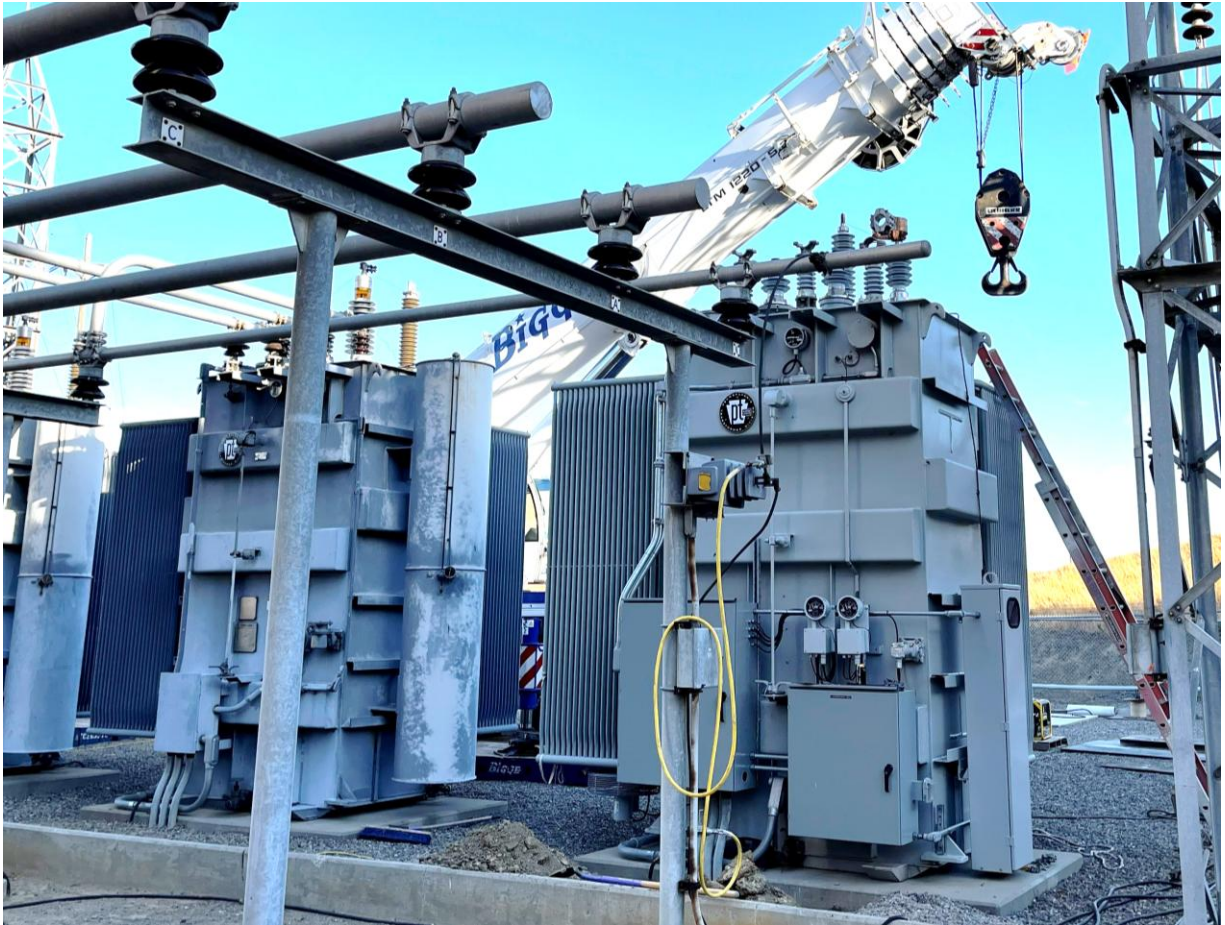
Existing 1960s Transformer (left) and Retrofilled/Rehabilitated Transformer (right) Figure 3
