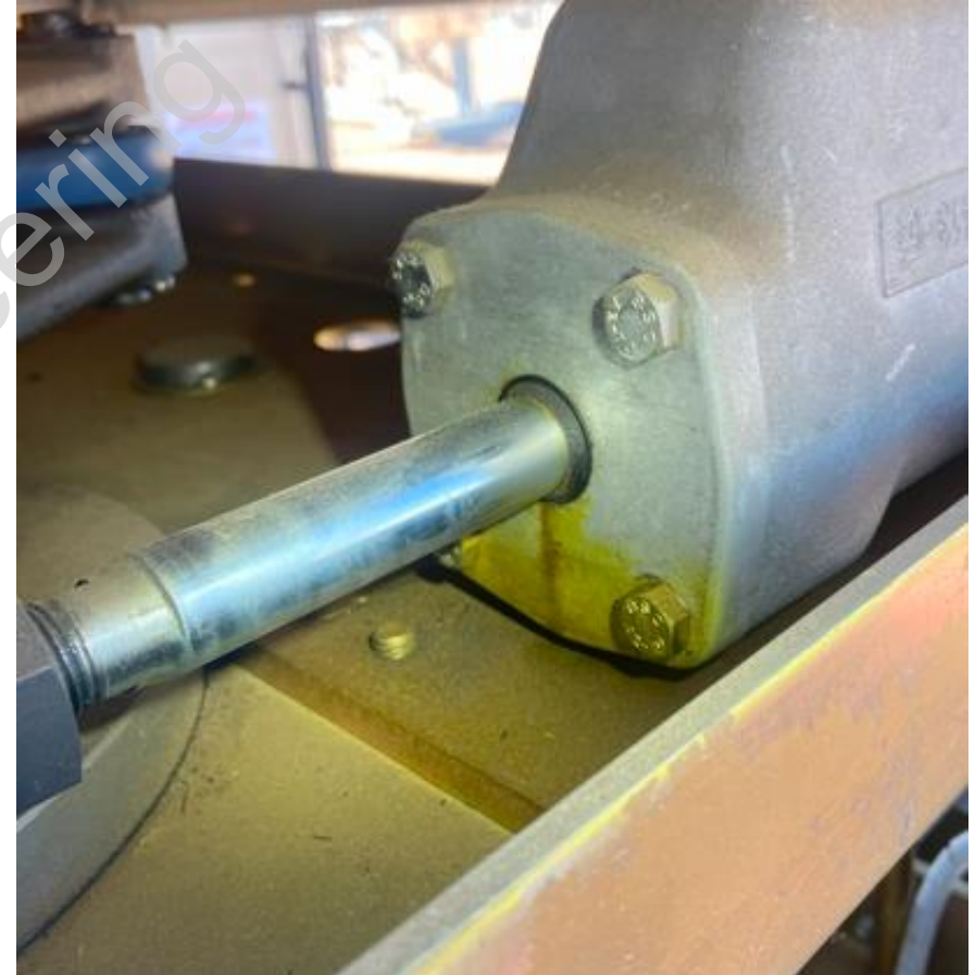
Signs of Leakage
