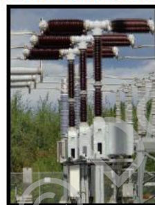
Live-Tank Breaker type HGF 100 series
