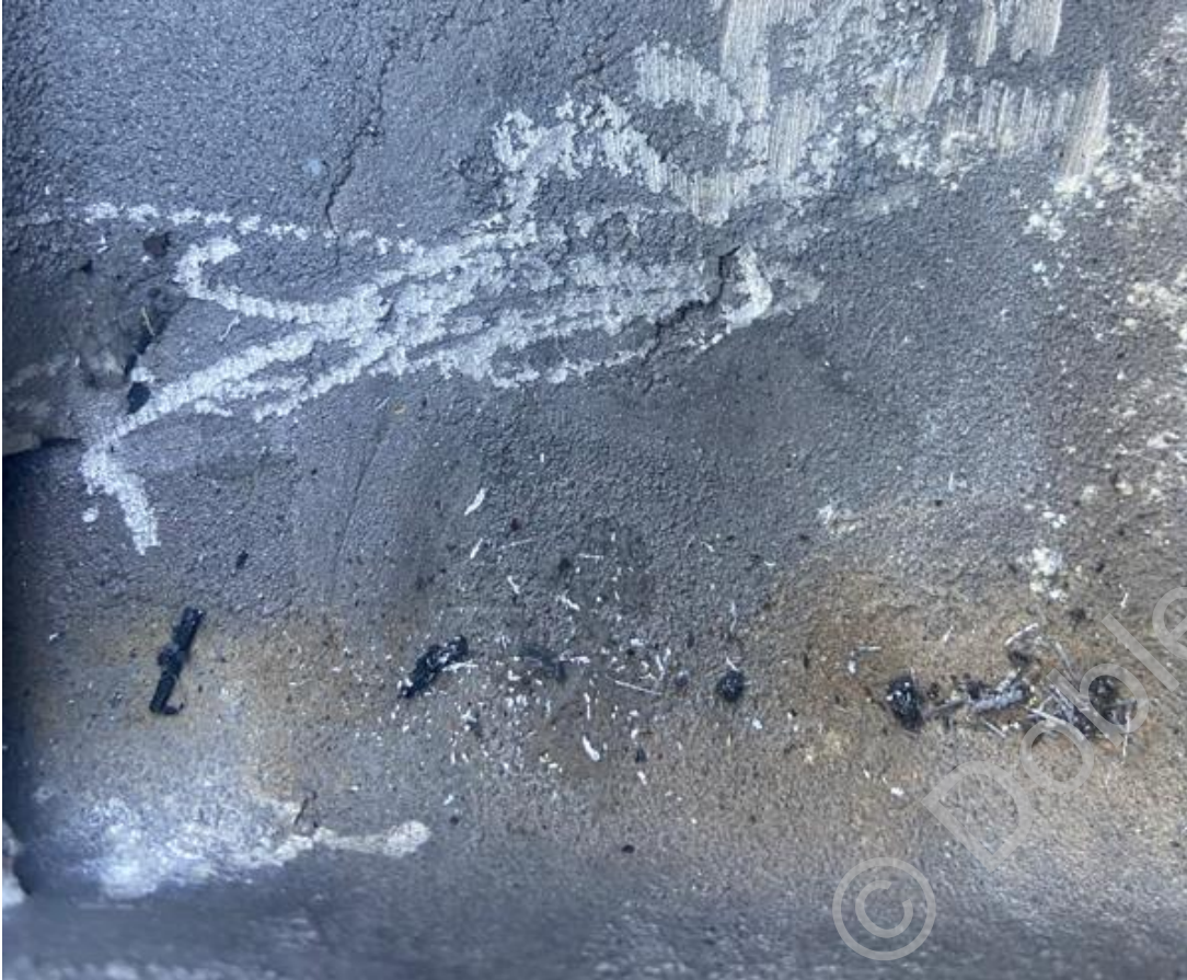
Significant metal shavings
