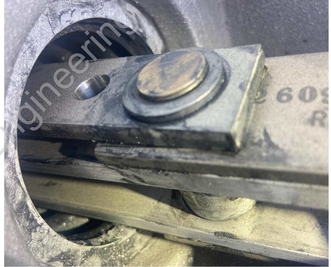
Linkage bent and scraping housing
