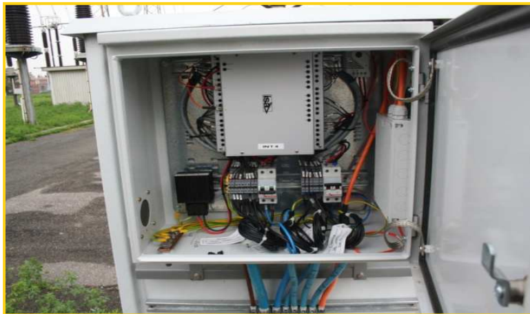
Figure 3 - Example of CB Monitoring installation
