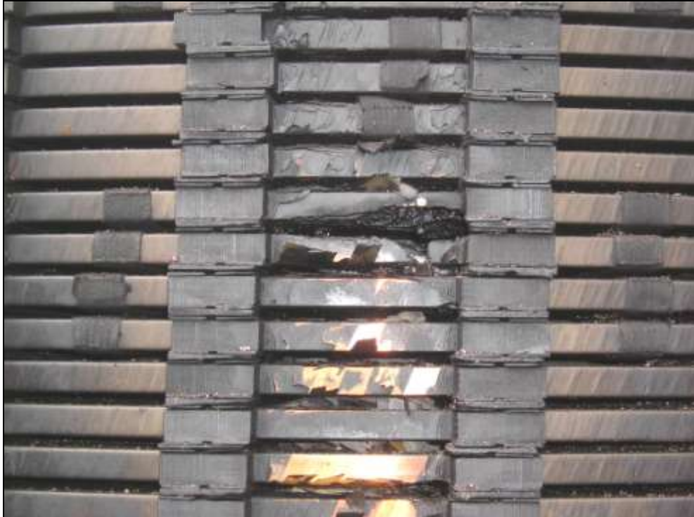
Case Study 2 – Consequential Damage to B Phase HV Winding, Close-up FIGURE 9
