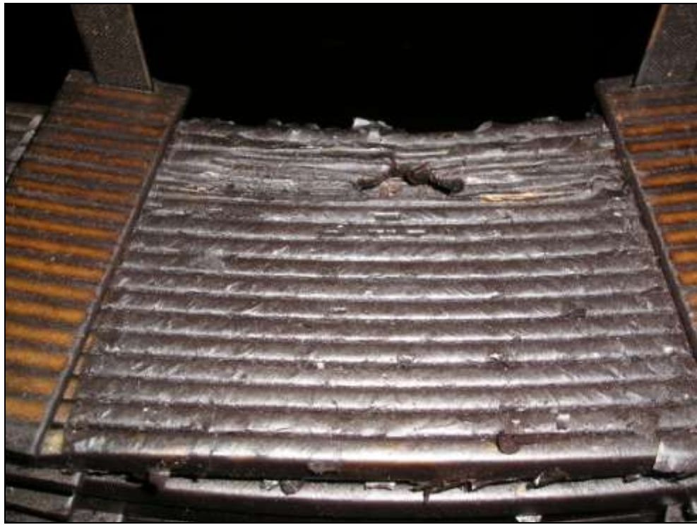
Case Study 3 – Point-of-failure FIGURE 12
