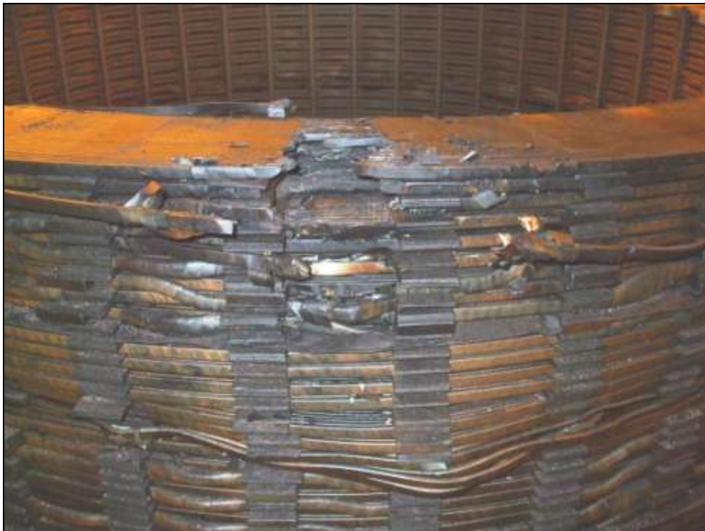
Case Study 1 – Damage to C Phase Series Winding, General View from Outside FIGURE 2
