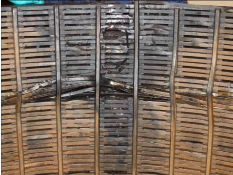
Case Study 1 – Damage to C Phase Series Winding, General View from Inside FIGURE 1
