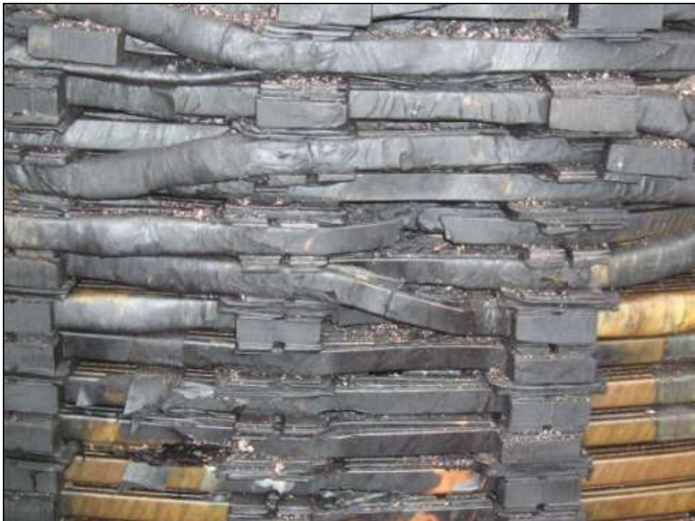
Case Study 2 – Damage to B Phase HV Winding, Close-up FIGURE 8
