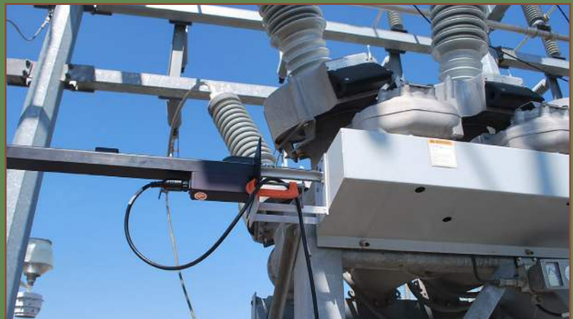
25" transducer on Siemens SPS2 Breaker
